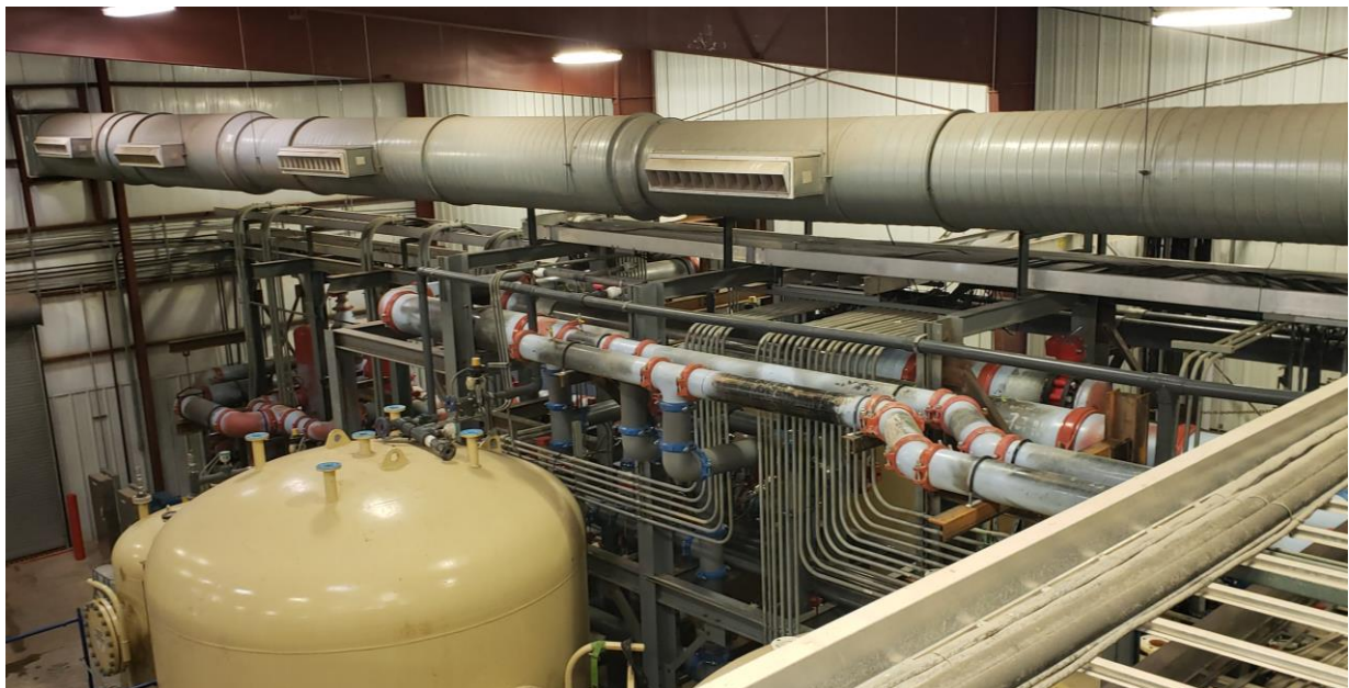
Figure 2 – Modified piping systems within the Ross Plant-Lance
