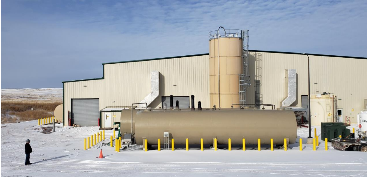
Figure 1 – The new acid storage vessels at the Ross Plant-Lance
