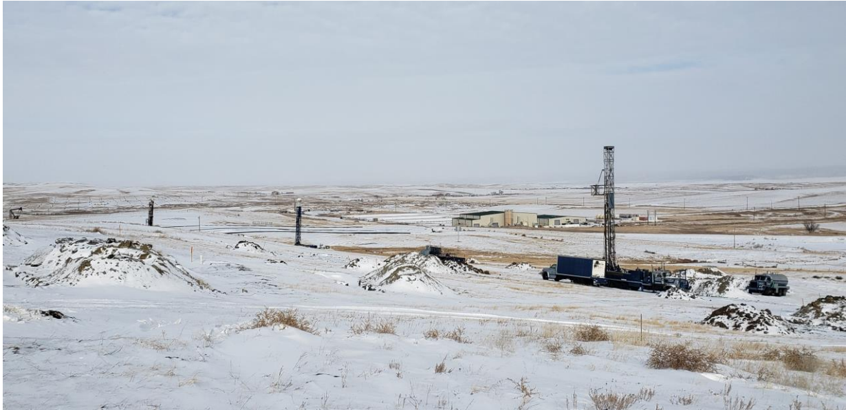
Figure 5– Multiple drill rigs working within MU-3 area. The Ross plant facilities are seen in the background
