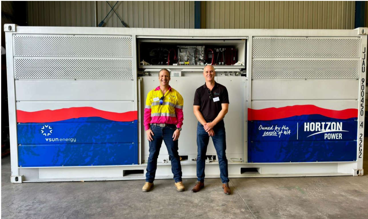
Figure 3 - AVL's Chief Safety & People Officer, Ross Jennings and VSUN Energy Manager, Zamien Sumich in front of the Horizon Power VFB
