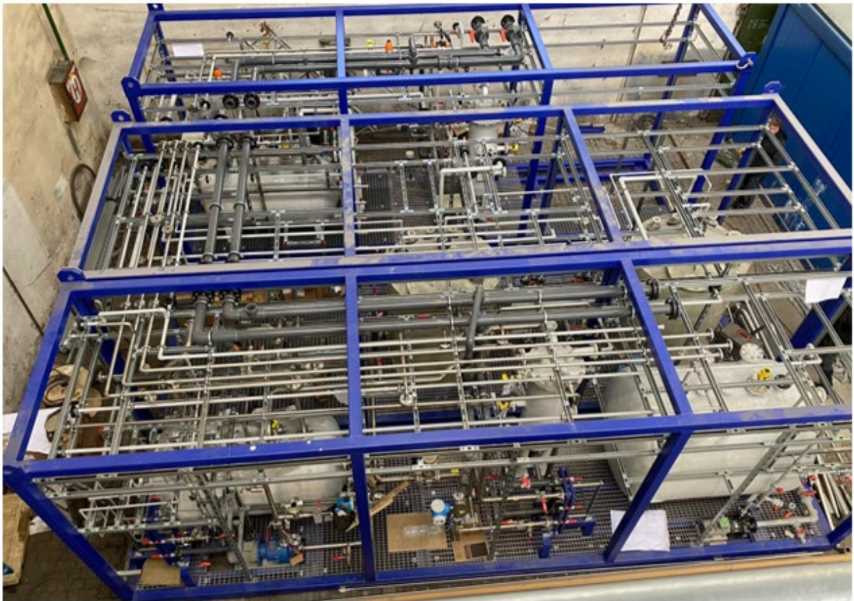
Figure 9 Electrolyser Equipment - Catholyte, Flushing & Anolyte
