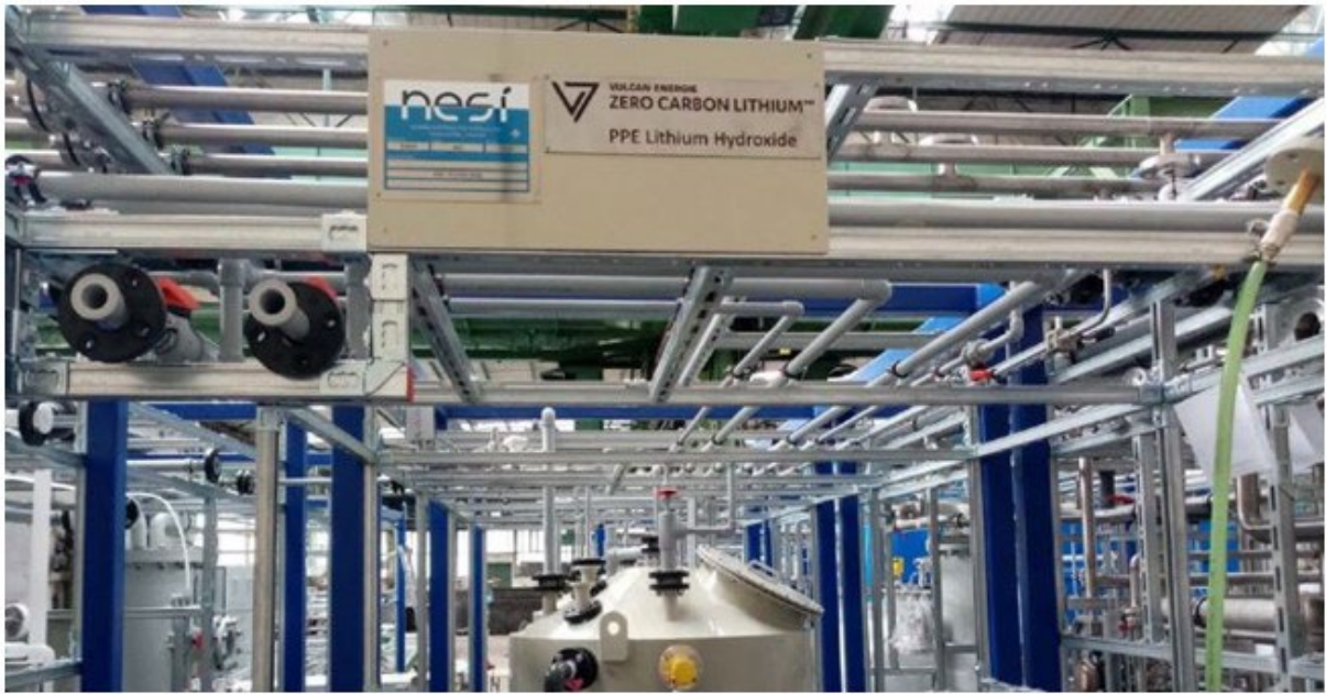
Figure 8 Electrolyser Equipment - Flushing (side view)
