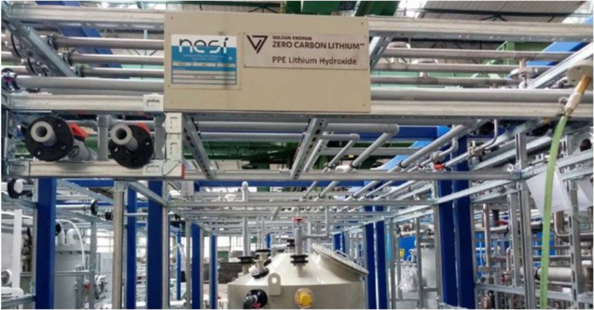
Figure 8 Electrolyser Equipment - Flushing (side view)
