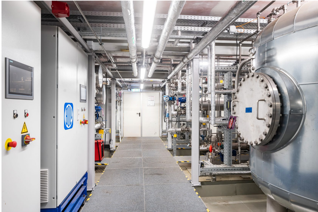
Figure 3 Inside the purification process room at Vulcan LEOP
