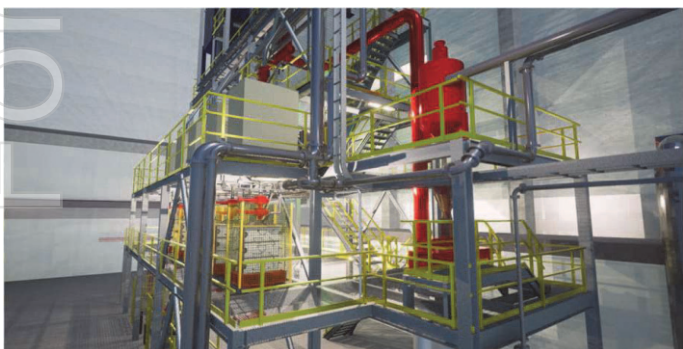
Figure 6: In-house designed packed bed calciners
