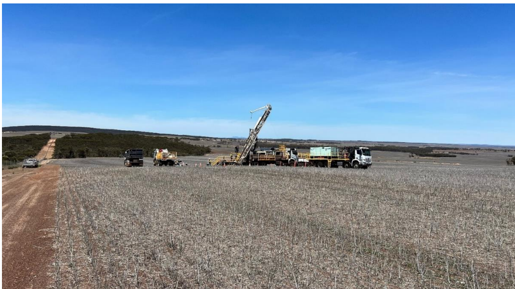
Figure 4: RC Drilling for lithium at the Ravensthorpe project, with Enviro Pod in use
