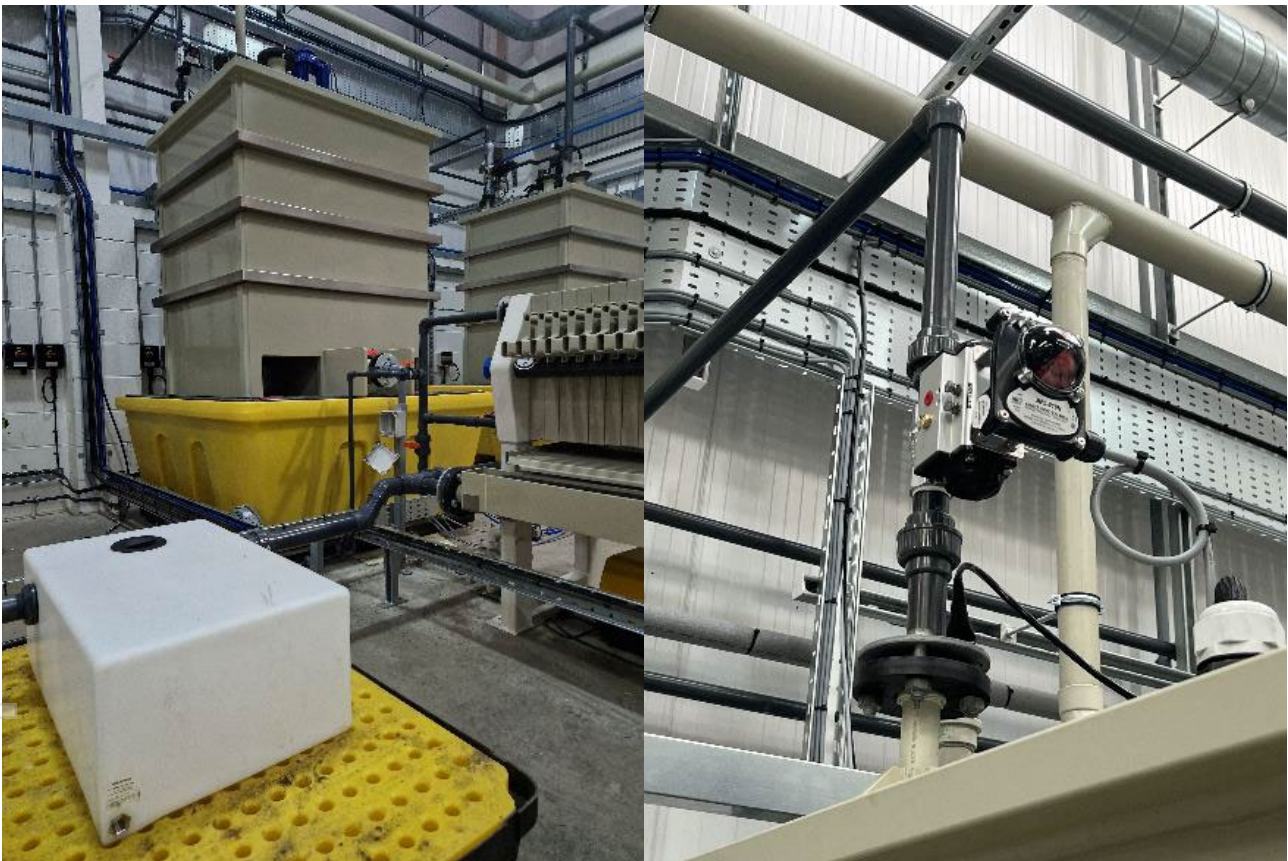
Figure 1: Reactor and Filter Press (shown in Figure 3 right) and automatic ball valve for feeding Reactor (right).
