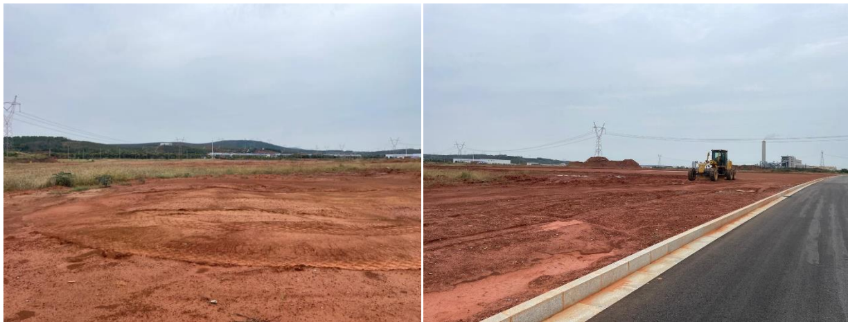
Image 2 and 3: Firebird's industrial land for its Sulphate Plant at Jinshi Chemical Park
