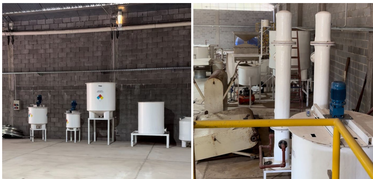
Figure 1 – Plant mixing tanks and columns being refurbished at the new Pursuit Lithium Facility in Salta, Argentina.
