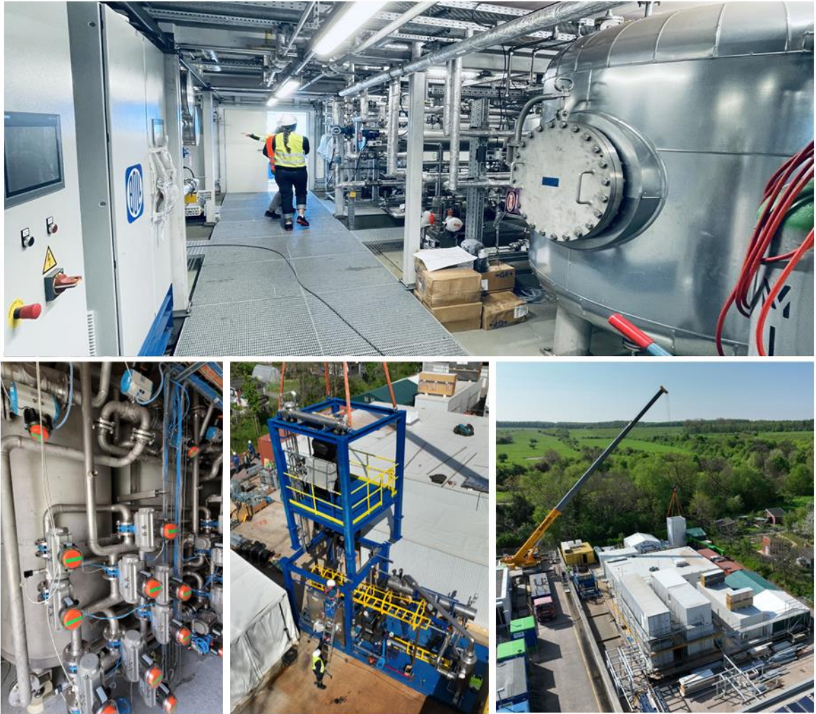
Figure 29 Vulcan's Lithium Extraction Optimisation Plant (LEOP).
