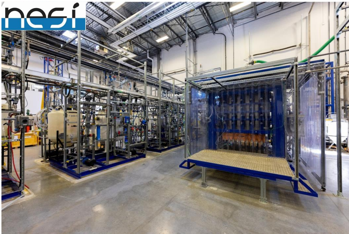
Figure 36 NORSCAND ® Cell Test setup at NESI's BC Research electrochemical demonstration plant facility in Vancouver.
