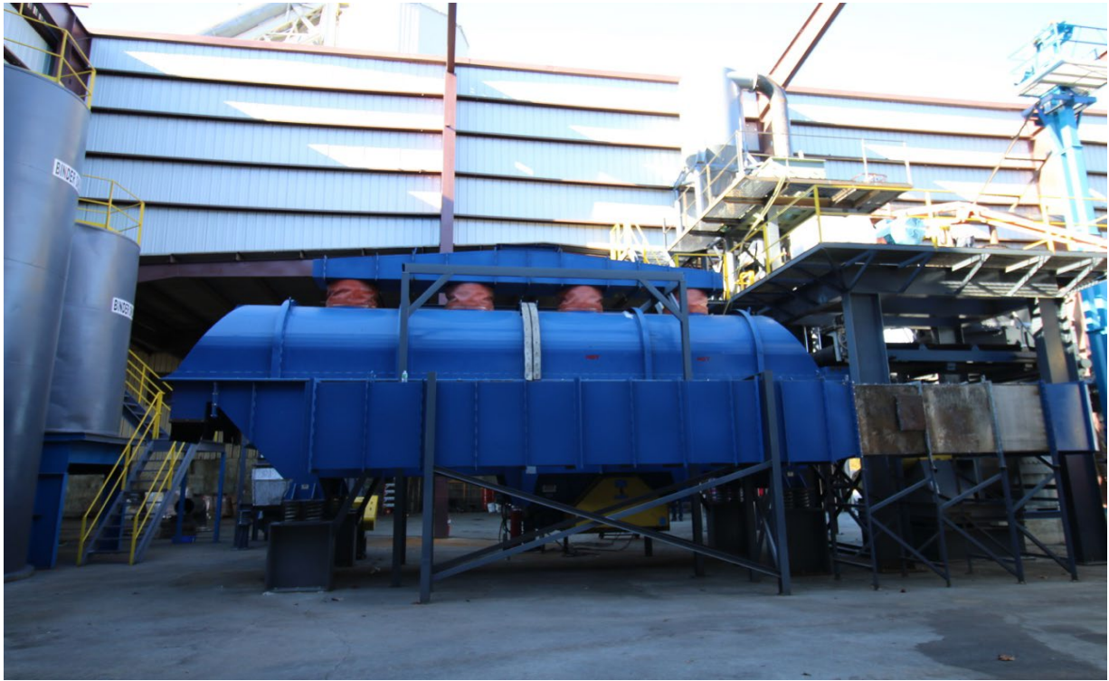
Figure 1: Drying and Baking
