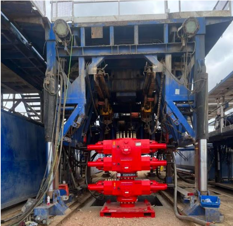
BOP and Sub-base of SLR 185 Rig
