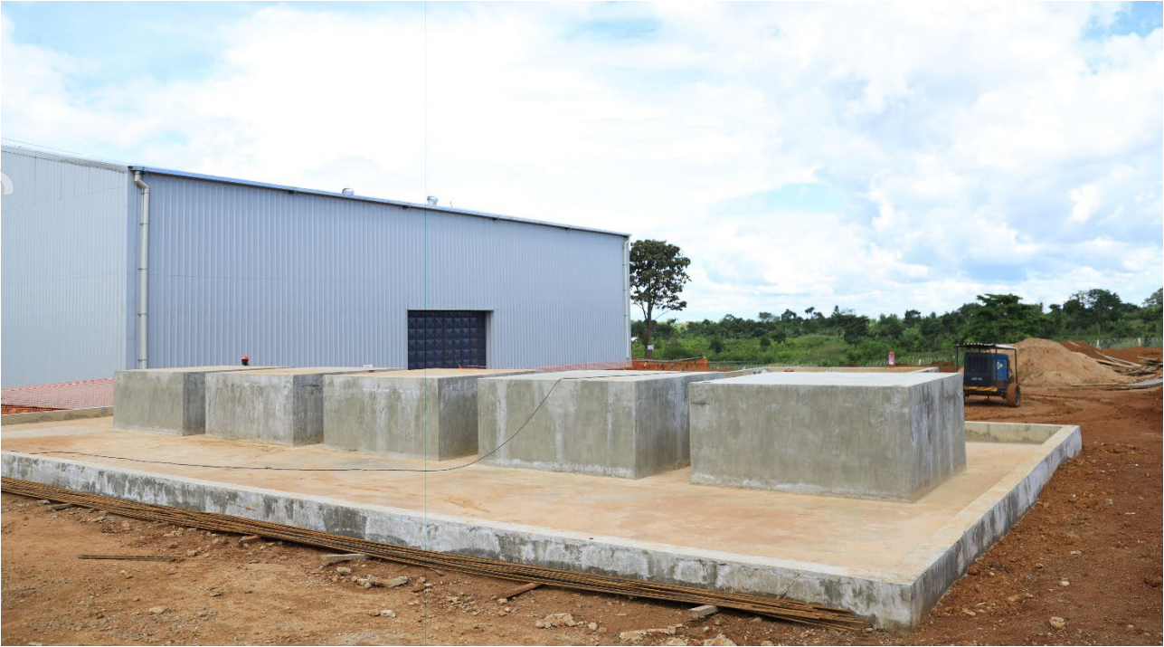
Figure 6: Makuutu Demonstration Plant Stage 1 desorption crib plinths, sump and bunded area.
