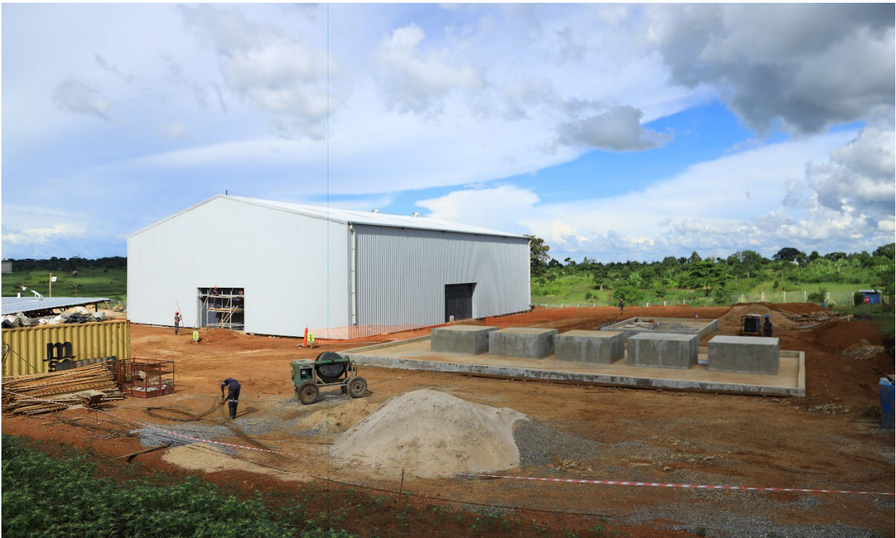
Figure 3: Makuutu Stage 1 Demonstration Plant with crib foundations in the foreground and Technical Facility in background.
