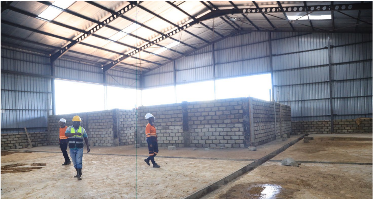
Figure 5: Technical Facility concrete slab, drains and sumps finalised and internal laboratory and office brickwork underway.
