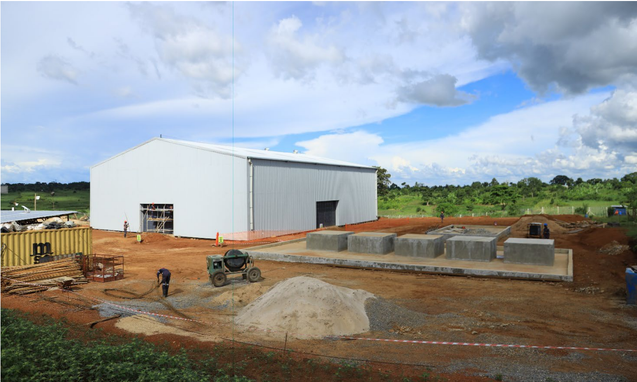
Figure 3: Makuutu Stage 1 Demonstration Plant with crib foundations in the foreground and Technical Facility in background.
