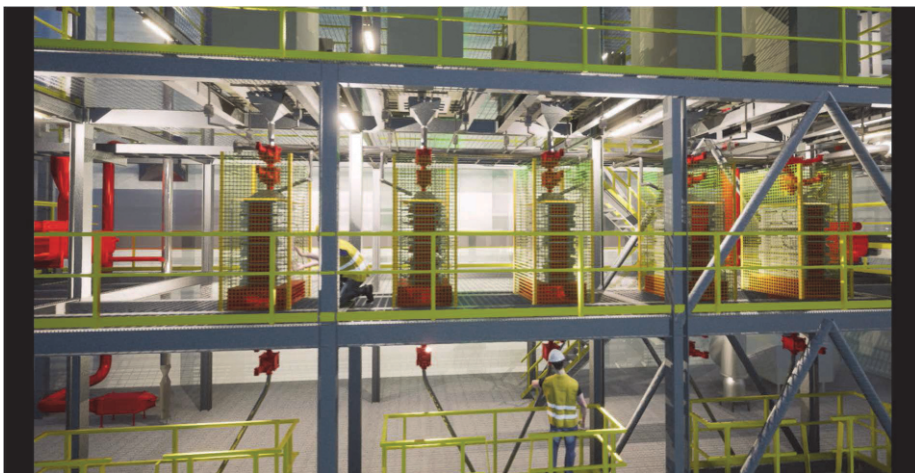
Packed bed calciners designed in-house
