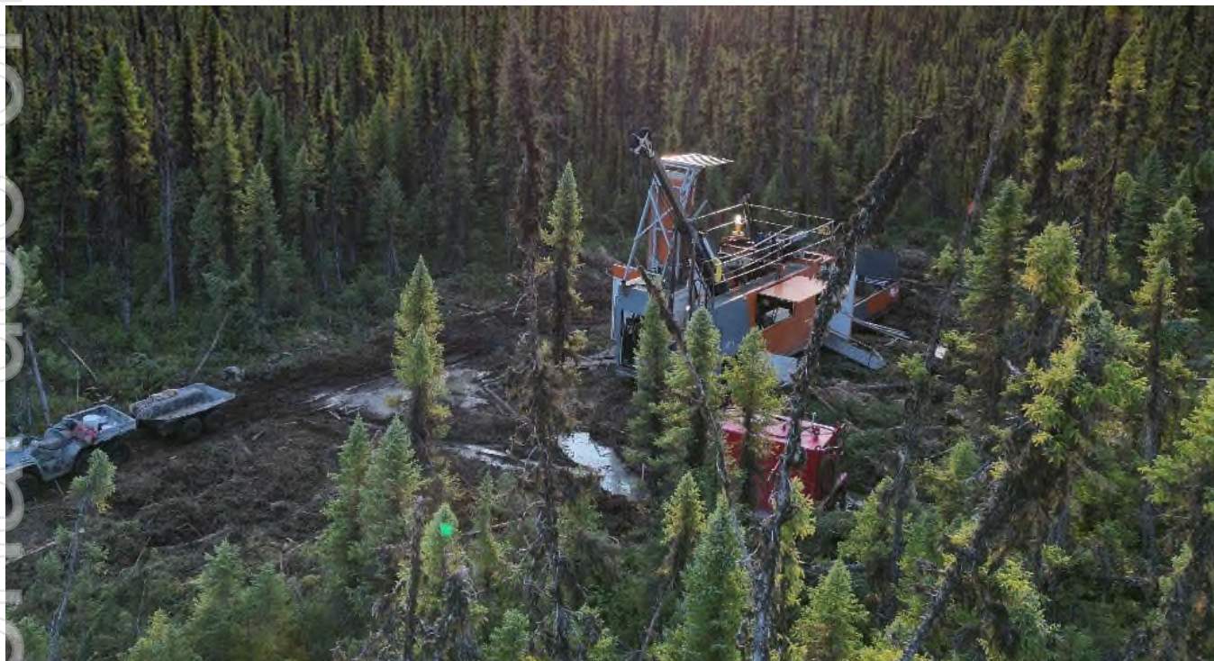
Figure 2: Diamond drill rig operational on hole POM-23-13 at the Pomme project, August 2023.
