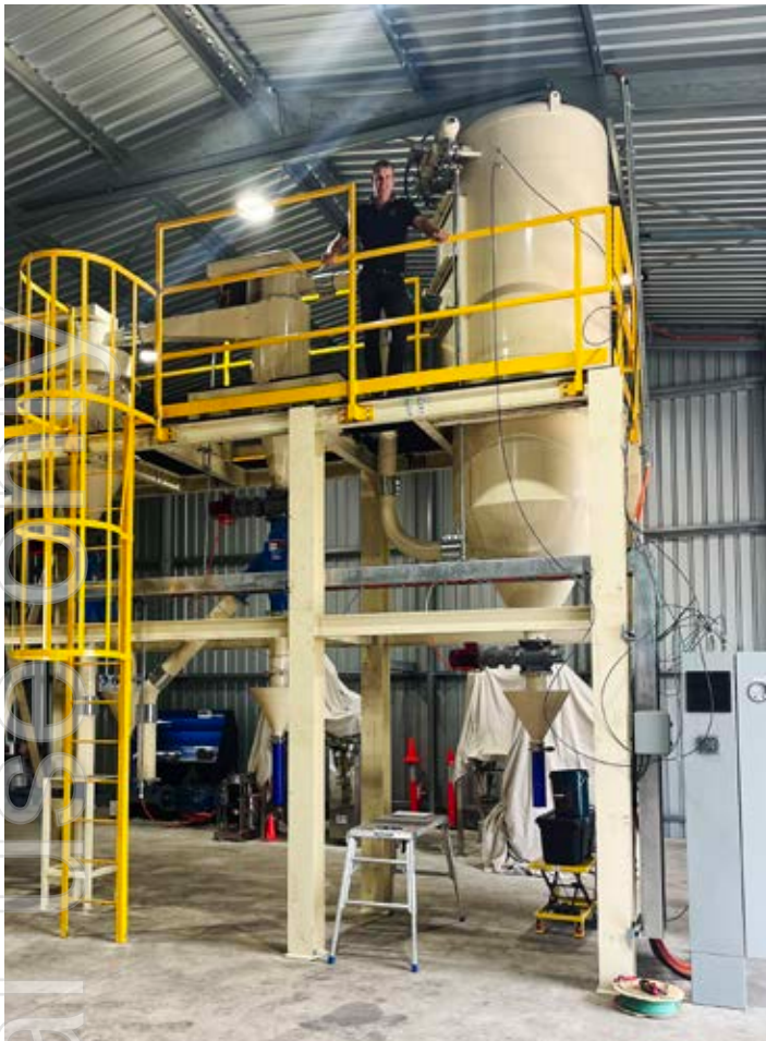
Figure 5: Qualification plant installation at International Graphite's R&D facility, in Collie, Western Australia.
