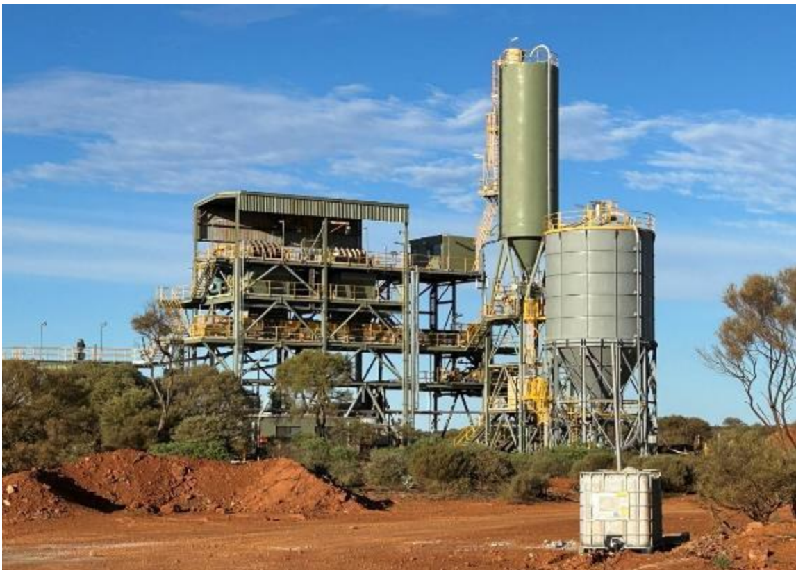
Figure 9 – Abra paste-fill plant.
