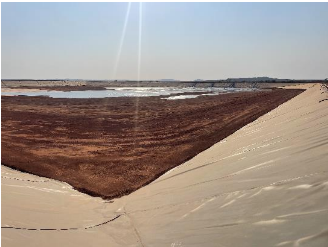
Figure 11 – Abra TSF Stage 1B (photo 23 October 2023).
