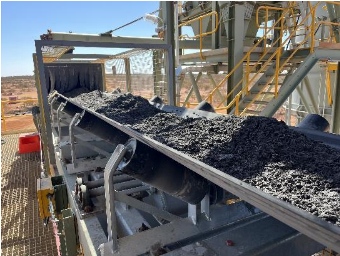
Figure 10 – Picture showing paste cake on the Abra paste-fill plant feed belt to the paste mixture (photo 4 October 2023).
