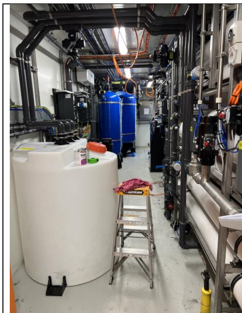
Image 1) De.mem Containerized Membrane Based Water Treatment Plant
