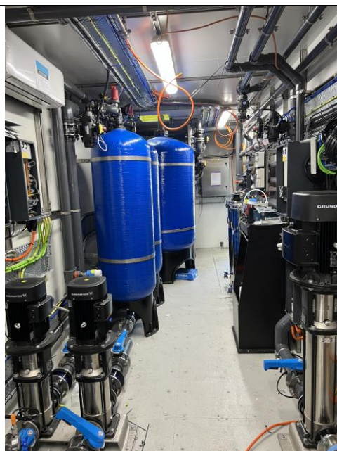
Image 2) De.mem Containerized Membrane Based Water Treatment Plant
