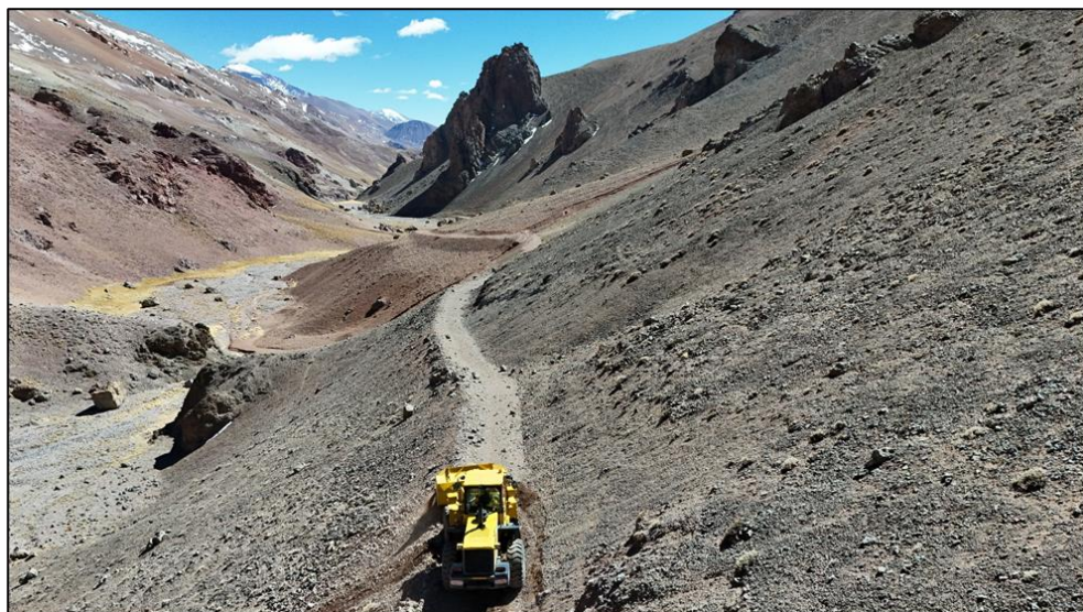
Figure 7: Drone shot capturing the restoration of the access track, track condition is prior to the first pass light vehicle upgrade works.
