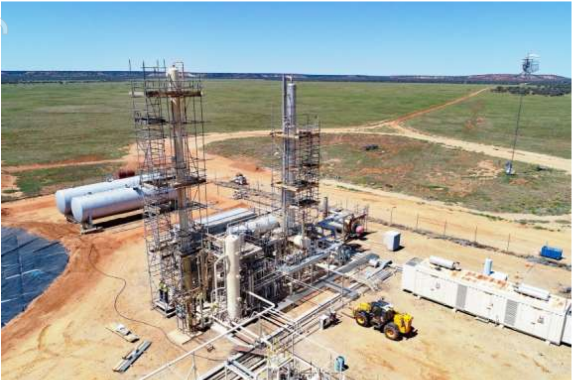
Eromanga Gas Plant
