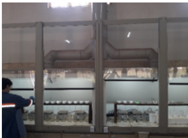
Fig 13 New exhaust system
