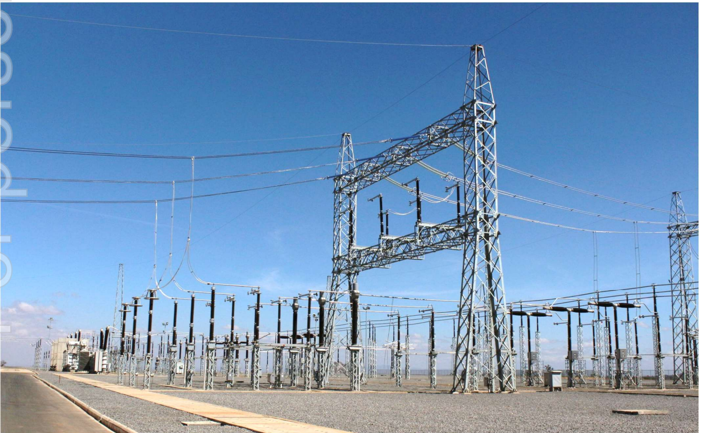
Figure 33: Nkhoma substation equipped for connection to the Kasiya operation
