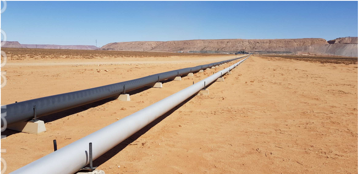
Figure 11: Example of overland pipes the concept planned for Kasiya (Source: Paterson & Cooke)
