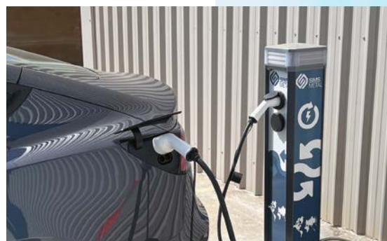
EV Charger at Sims Metal Kwinana
