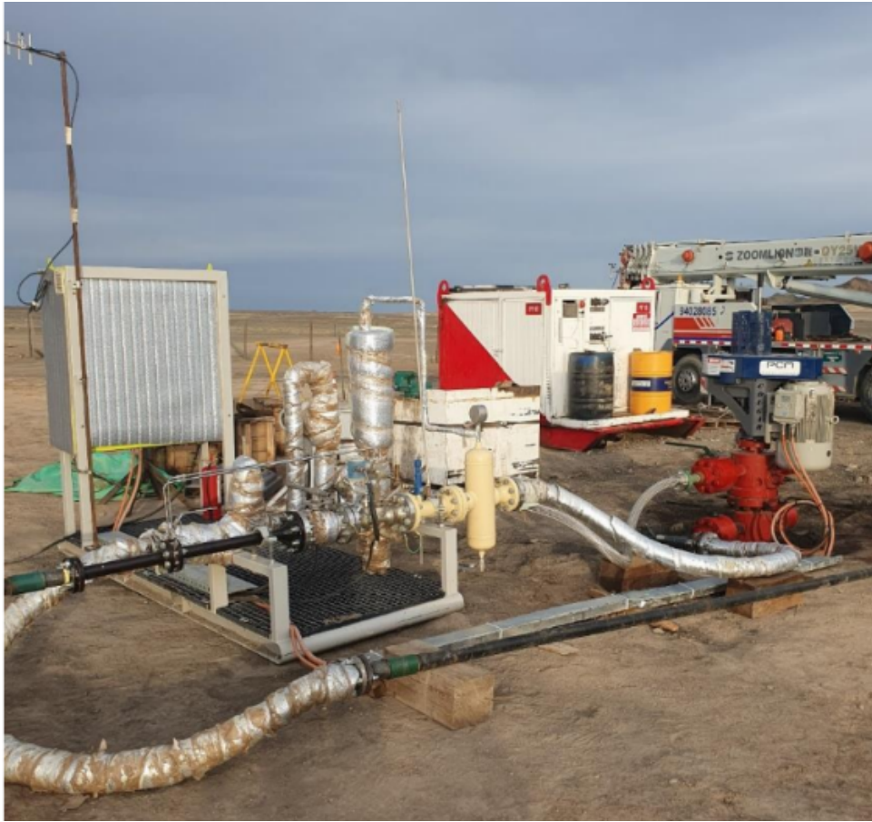
Nomgon-10 Production Skid
