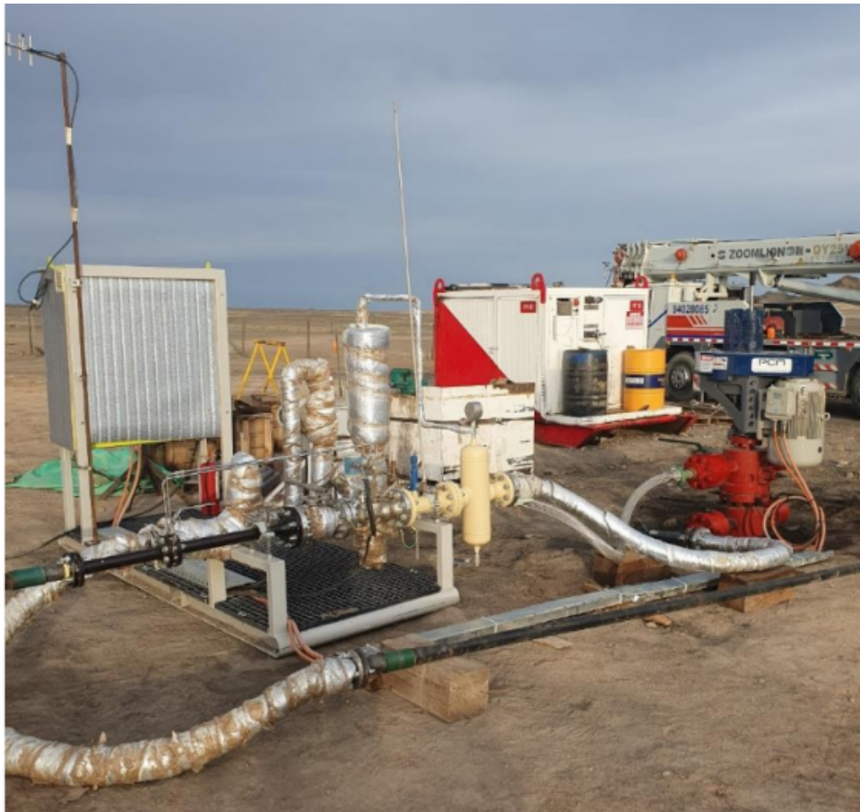
Nomgon-10 Production Skid
