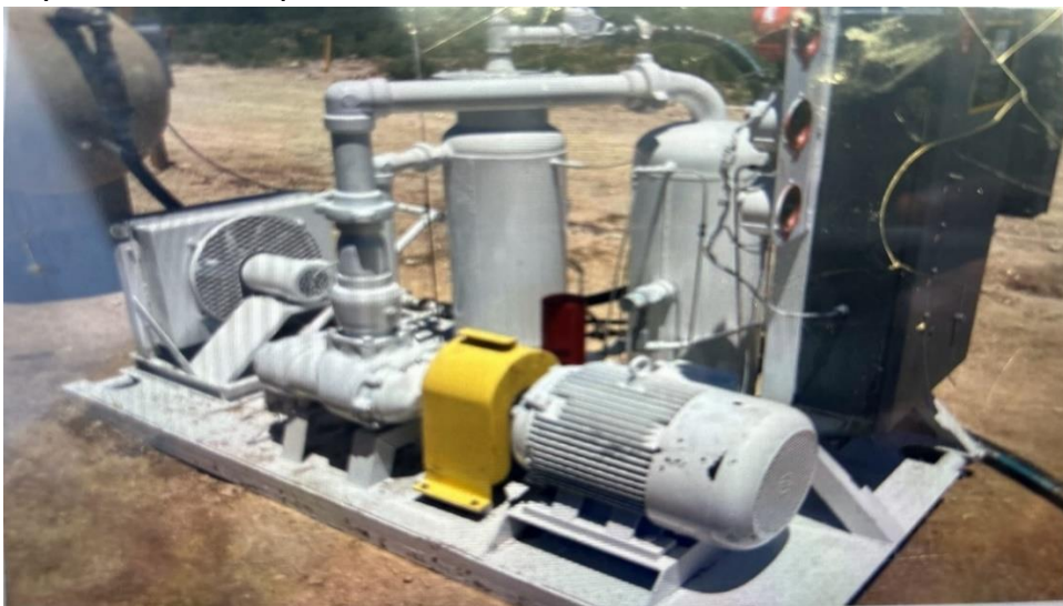
Figure 2: Electrically Driven “Smart Compressor” Installed at White Hat Ranch
