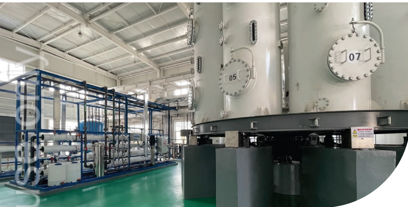
Figure 3: Lanshen DLE test facility in Xian, China
