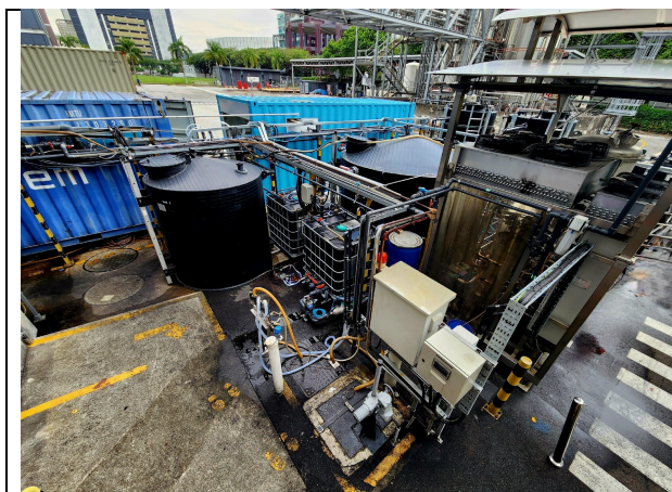
Image 1) De.mem Singapore BOO waste water treatment plant
