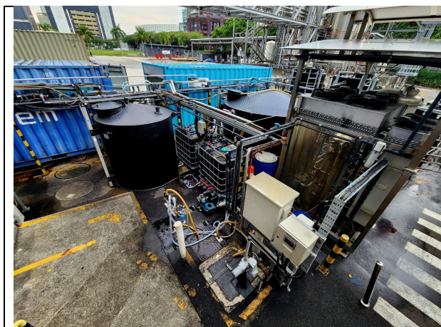
Image 1) De.mem Singapore BOO waste water treatment plant
