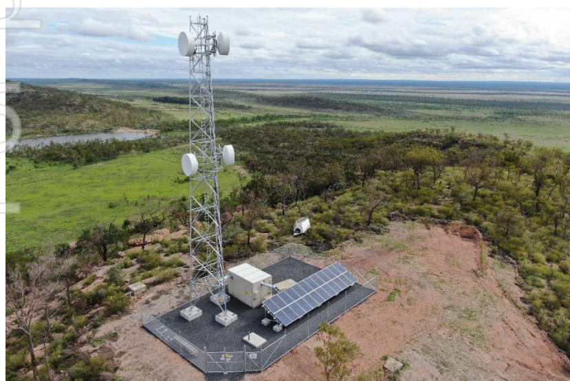
1 High-capacity wireless telecommunication installation in Queensland
