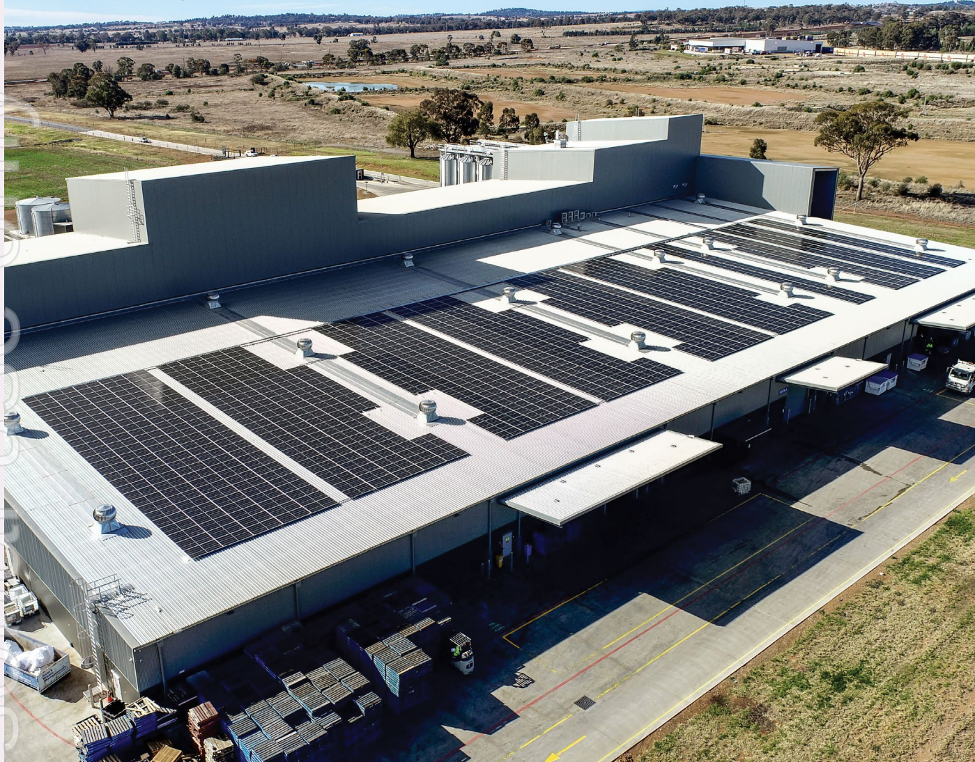
Roof-mounted solar array at Parkes, NSW
