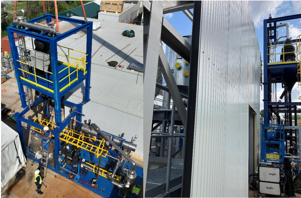
Figure 2 and 3. Crystalliser installation
