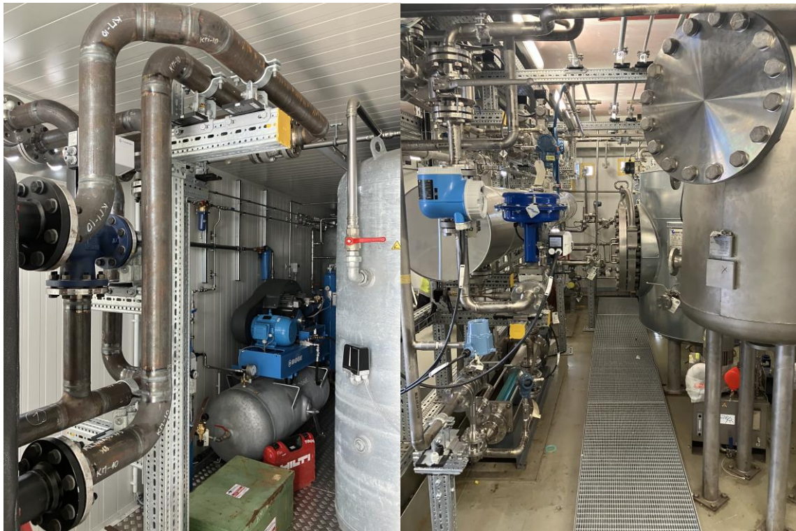
Figure 4. Utilities nitrogen and cooling water
