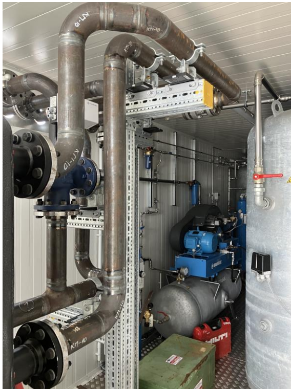
Figure 4. Utilities nitrogen and cooling water
