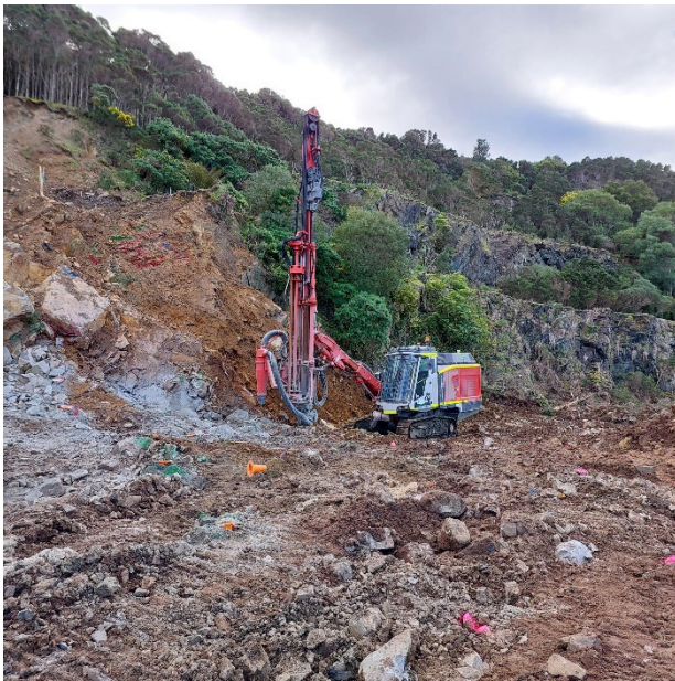
Figure 2 - Drilling ongoing in "West Pit" on western side of Dolphin Open Cut
