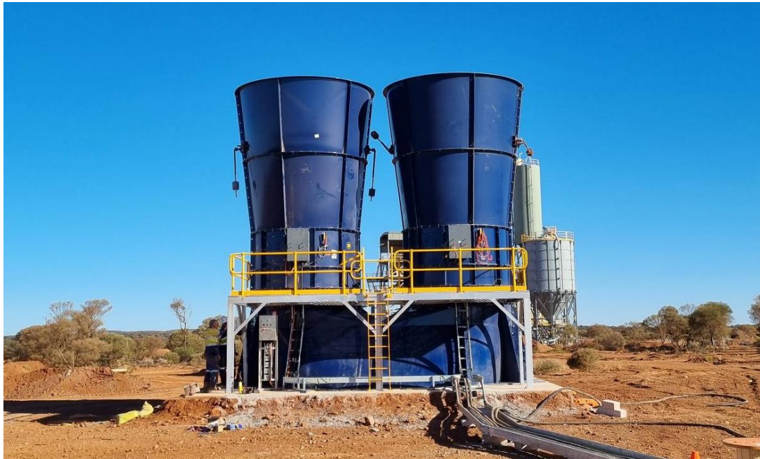
Figure 2 – Successful installation of the second primary ventilation fan at Abra during July on the mine’s primary 6m diameter exhaust rise (Photo 25 July 2023).
