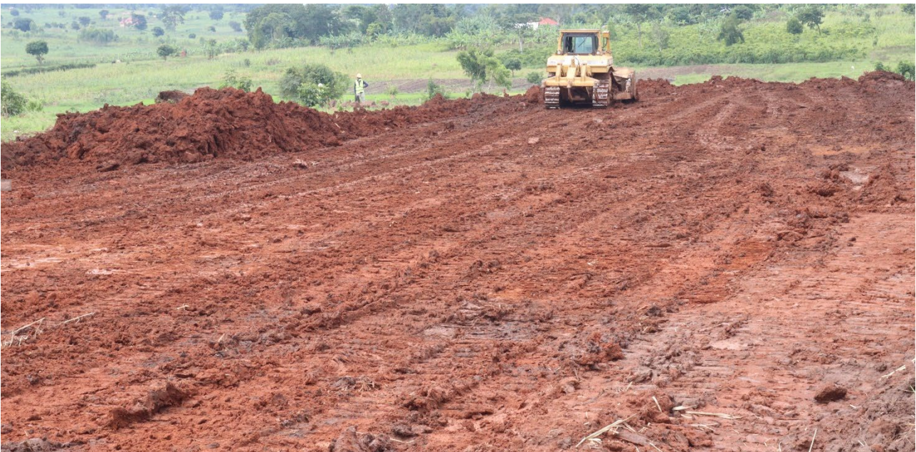
Figure 2: Demonstration plant earthworks progressing at the site of where the Makuutu Demonstration Plant Technical Facility will be located.
