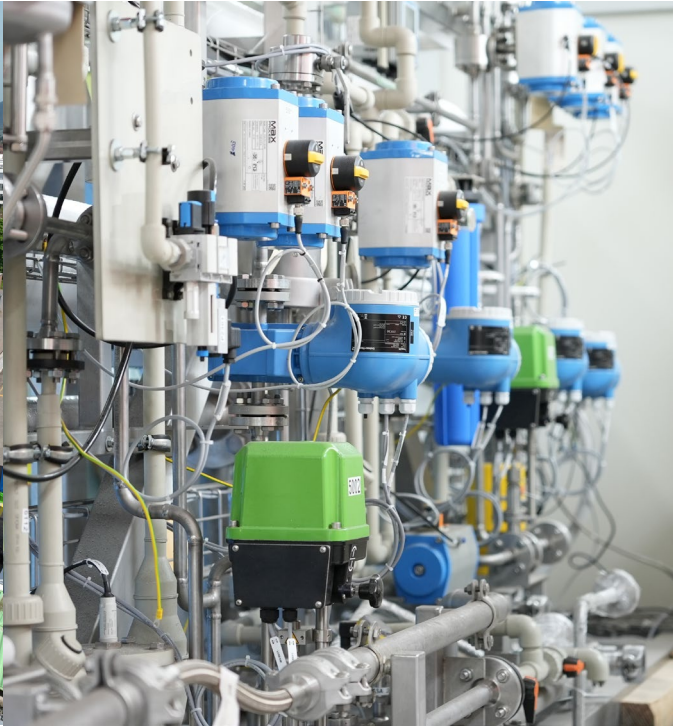
Figure 2 Electrical installation LEOP, Landau
