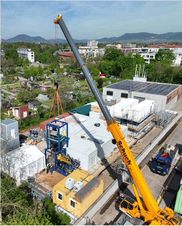
Figure 1 Installation of Crystallizer at LEOP, Landau
