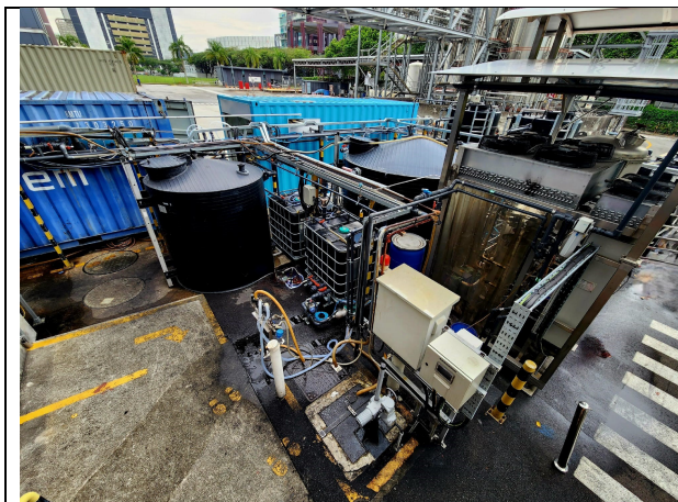
Image 1) De.mem Singapore BOO waste water treatment plant
