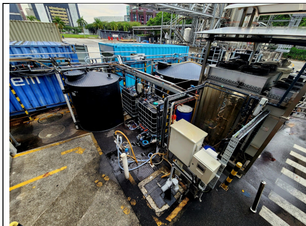
Image 1) De.mem Singapore BOO waste water treatment plant
