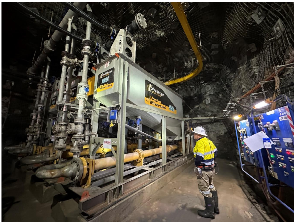
Figure 7 – Galena Managing Director, Tony James, inspecting the fully commissioned primary pumping station underground at Abra (Photo 13 July 2023).
