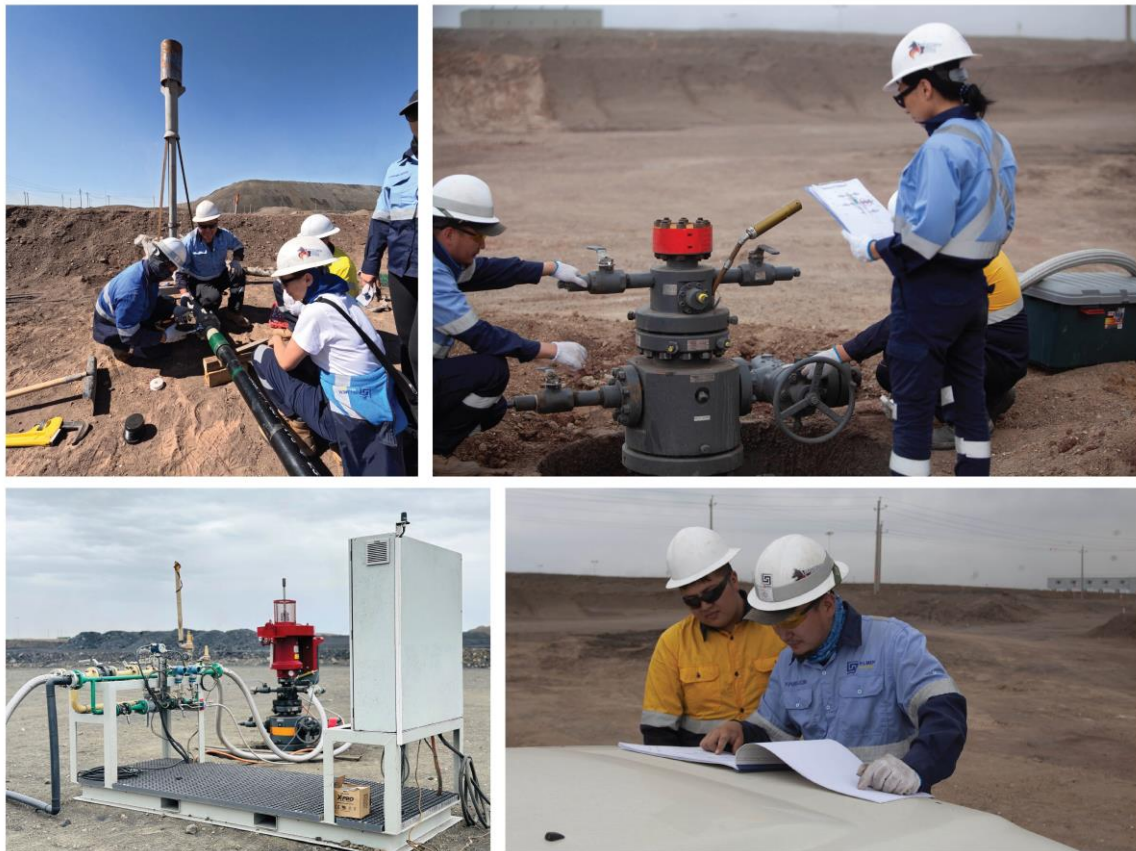
Figure 1 – Commissioning activities on the three production wells at the Pilot Well Program
