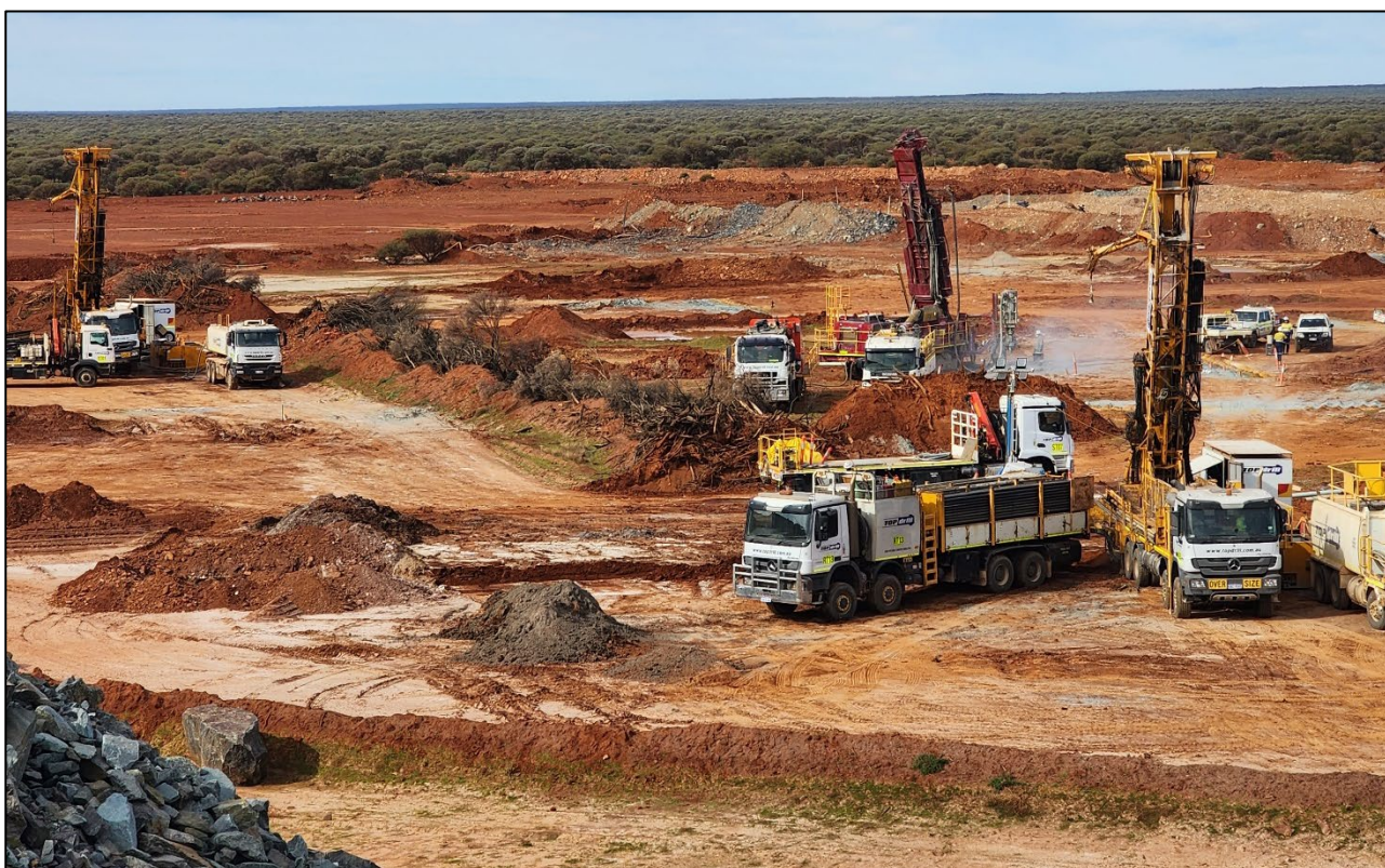
Figure 1: Never Never resource and extensional drilling campaign. Three rigs operating within DMIRS approved and cleared Never Never Open Pit mining footprint – June 2023.
