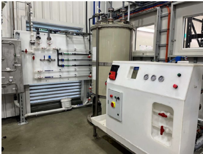
Figure: Crystallisation unit
