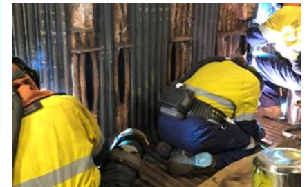
BOILER TUBE LEAD REDUCTION PROGRAM
