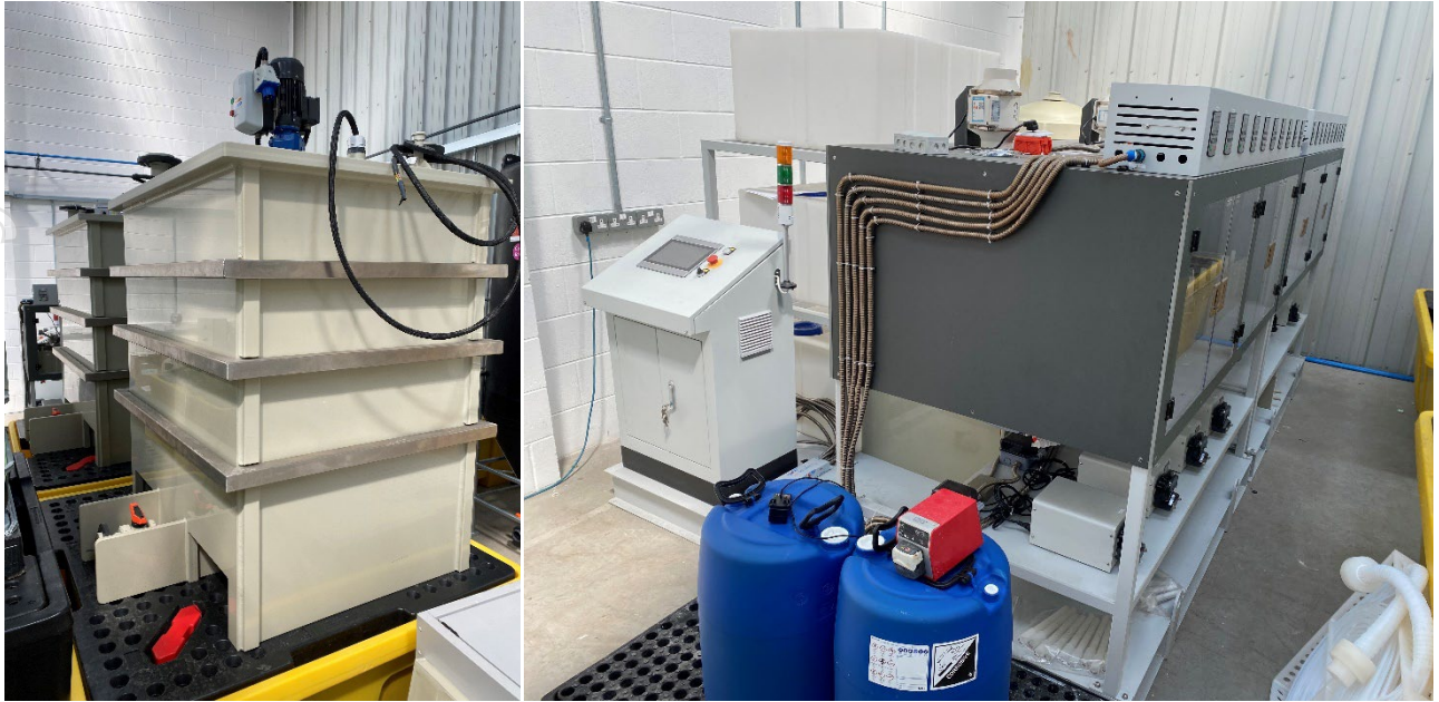
Figure 2: Leach reactors and Solvent Extraction circuit electrical installation completed, with process commissioning underway.
