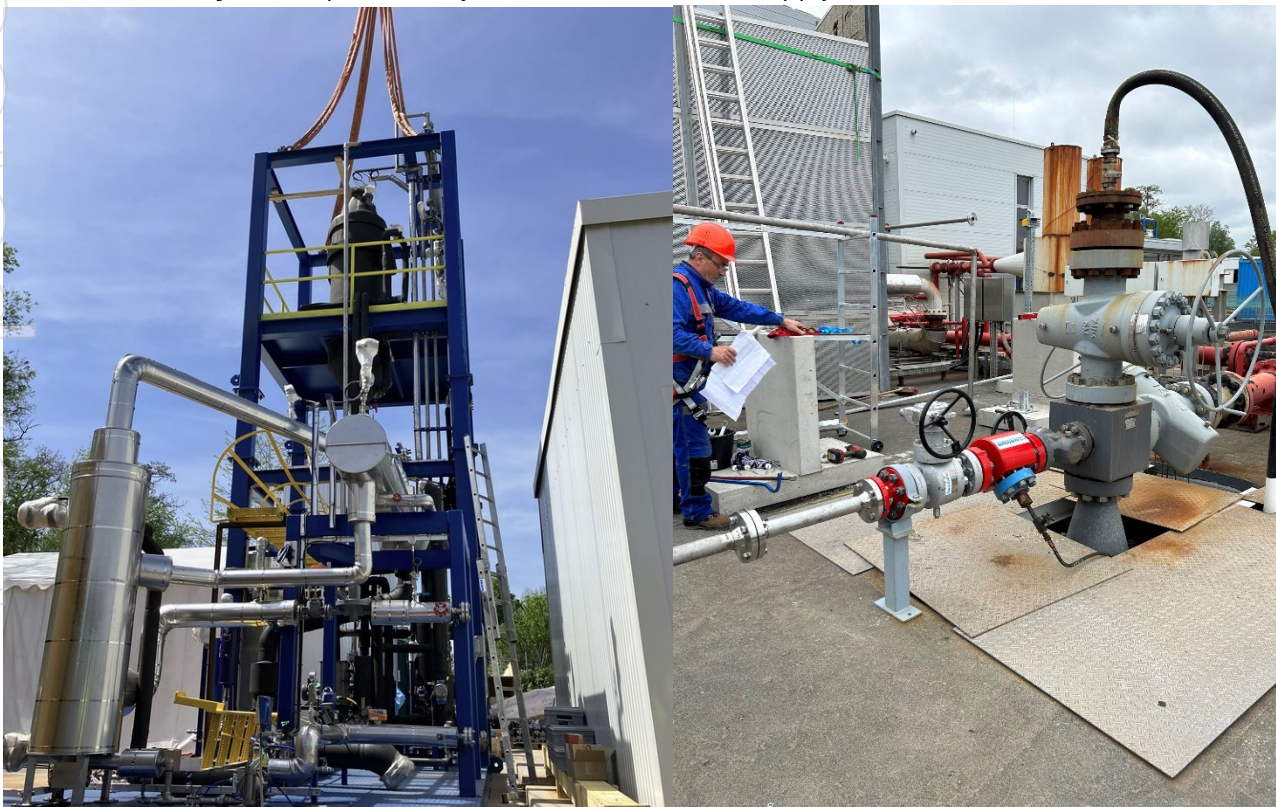
New crystallizer at Vulcan's Lithium Extraction Optimisation Plant
