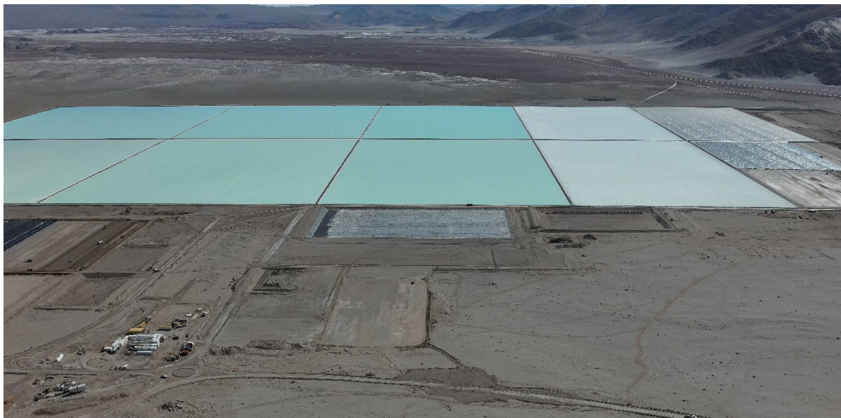
Figure 1: Sal de Vida Stage 1: First 2 string of ponds are 90% complete and carbonation plant development advances
