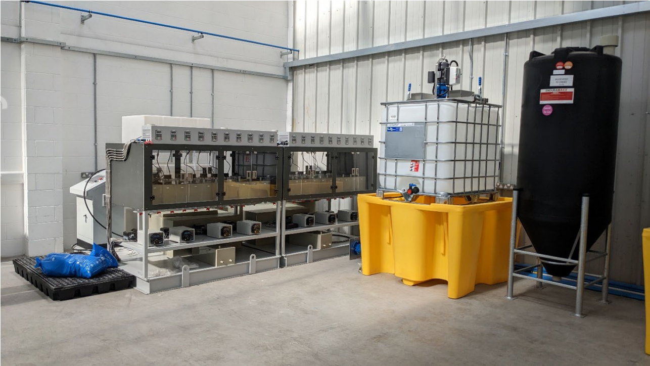
Figure 6: Mixer-Settler circuit installed adjacent to process reactor and settling tank.
