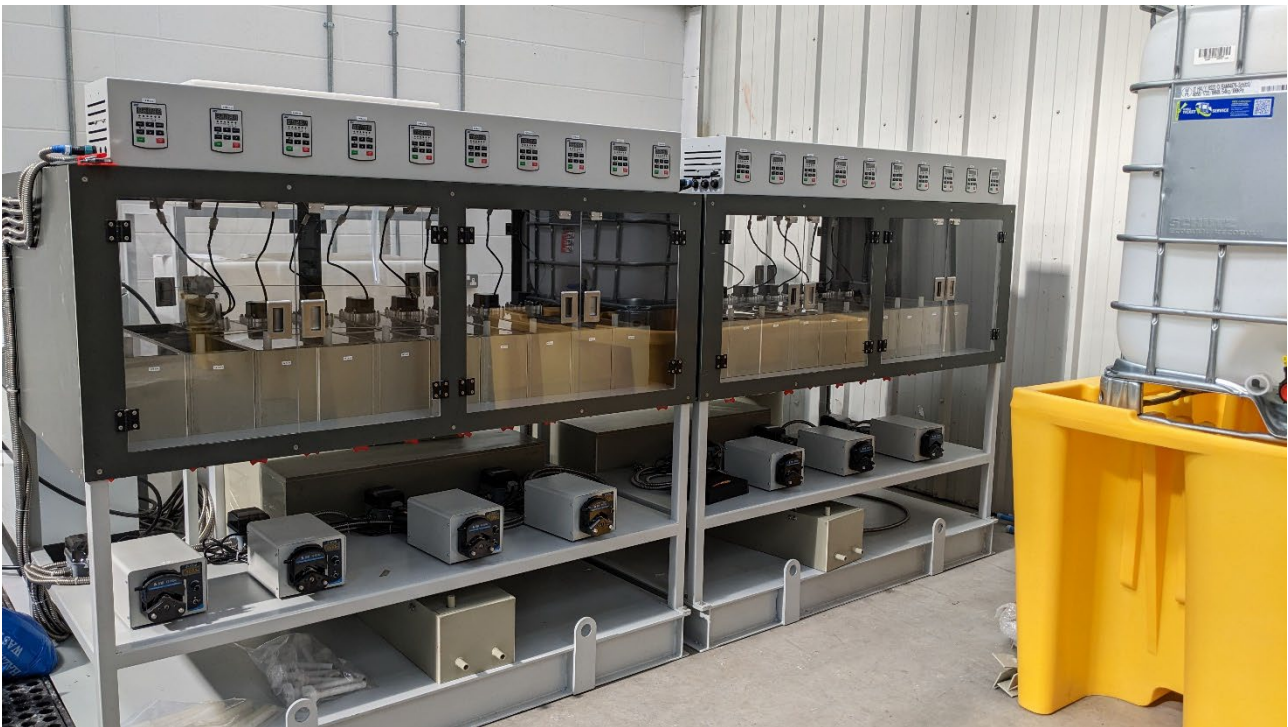
Figure 5: Mixer-Settler circuit installed.
