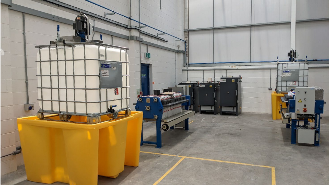
Figure 4: Plate and Frame filters in position along with process vessels and product drying kilns.
