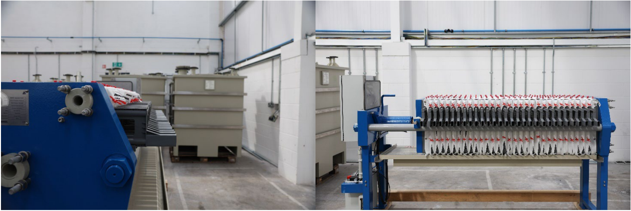
Figure 8: One of the Plate and Frame filter presses in position adjacent process reactor vessels.
