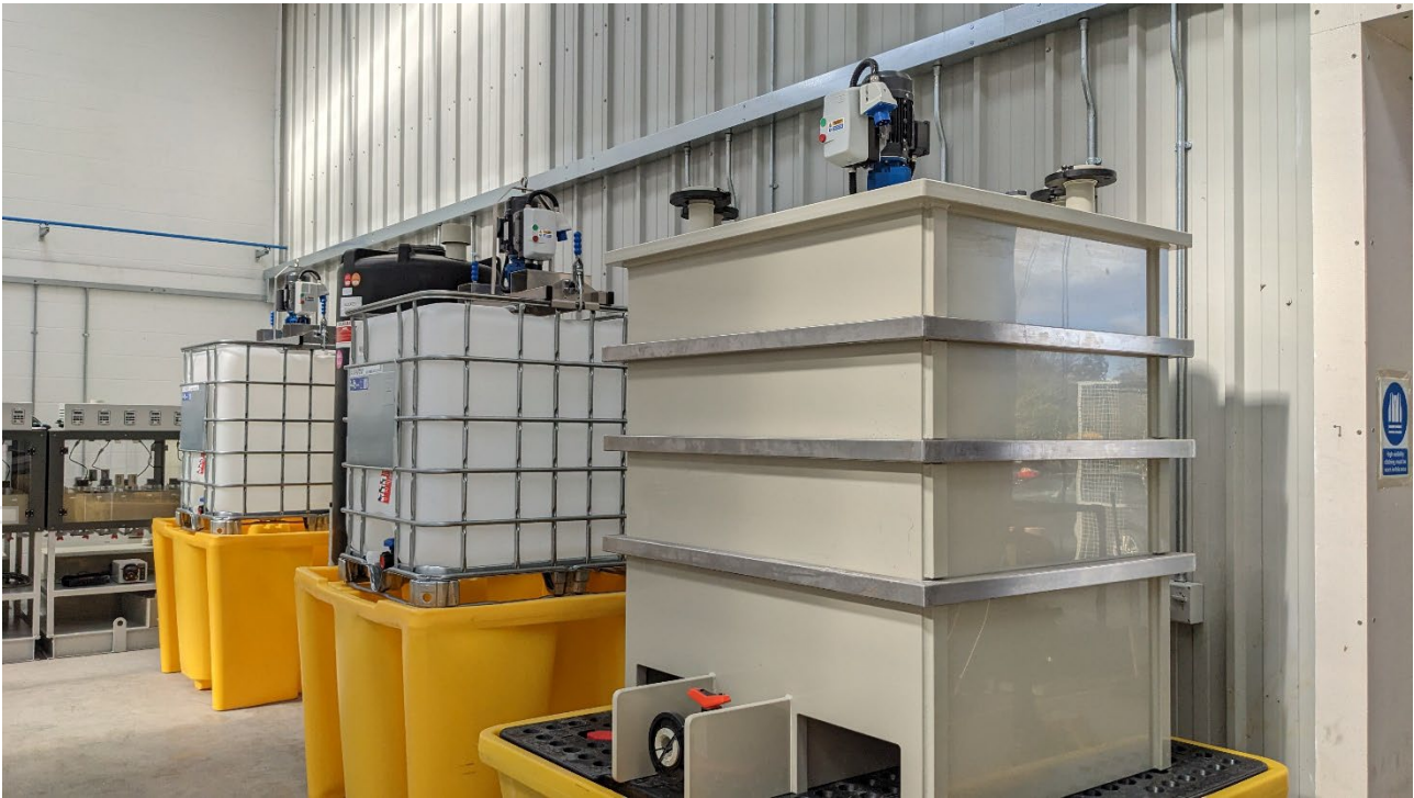
Figure 7: Process reactors installed in position adjacent mixer settler circuit.
