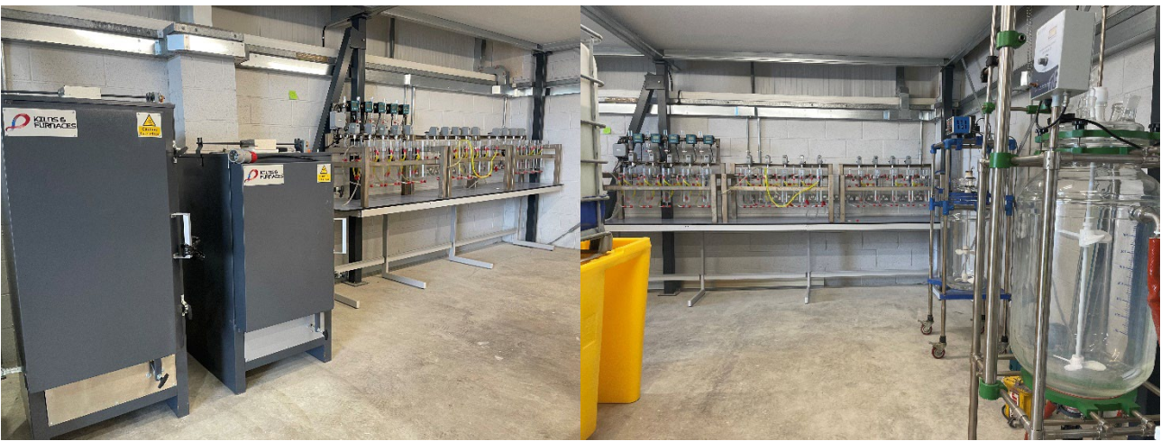
Figure 9: Pilot plant relocated to new mezzanine area; left, demagnetisation oven and product drying kilns, and right showing glass reactor arrangement adjacent mixer-settler circuit.
