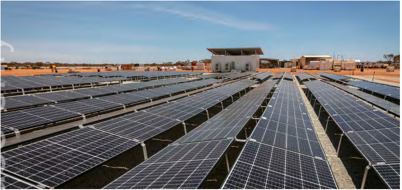
Picture Above Yamarna camp solar array
