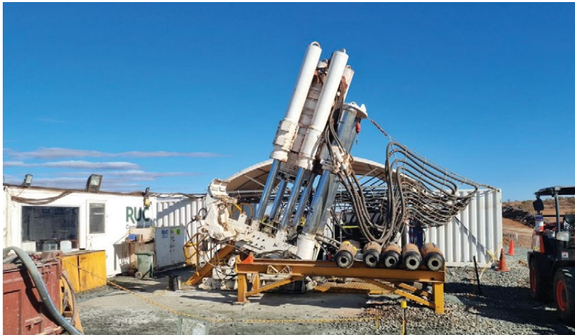
Figure 8: Bellevue site RUC raisebore drilling at the Northern escapeway rise (right); Second raisebore drilling rig at the Southern ventilation rise (below right)
