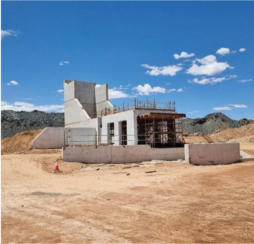
Figure 5: Construction progress on the Primary Crusher facility at the processing plant as at 24 January 2023
