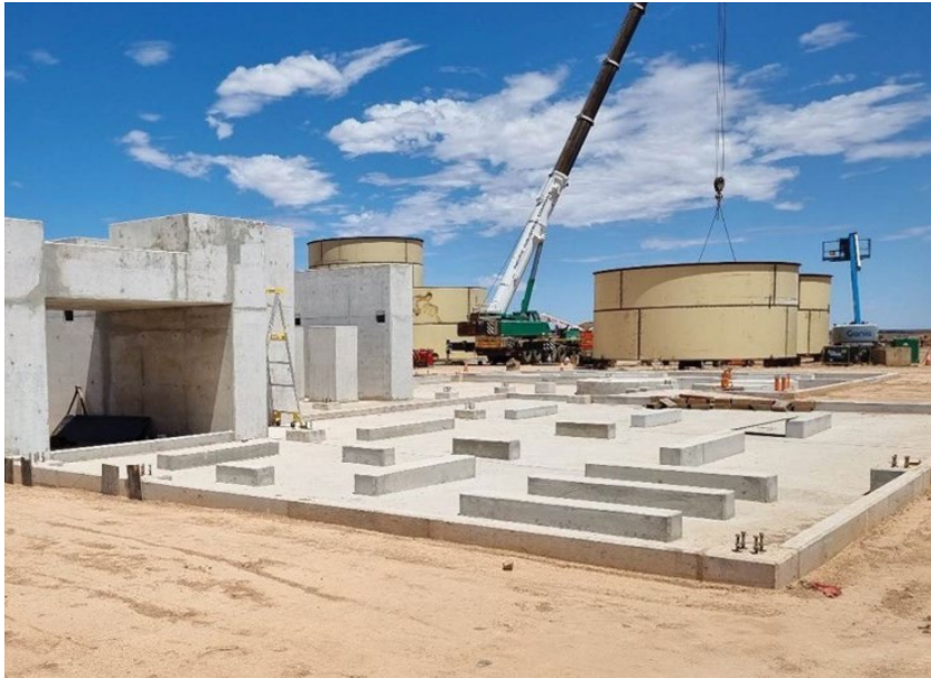
Figure 6: Construction progress on the ball mill foundations at the processing plant as at 24 January 2023
