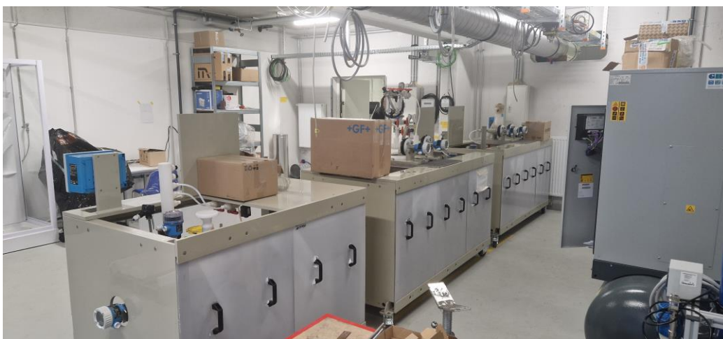
Figure 3 – Pilot Plant Test Equipment
