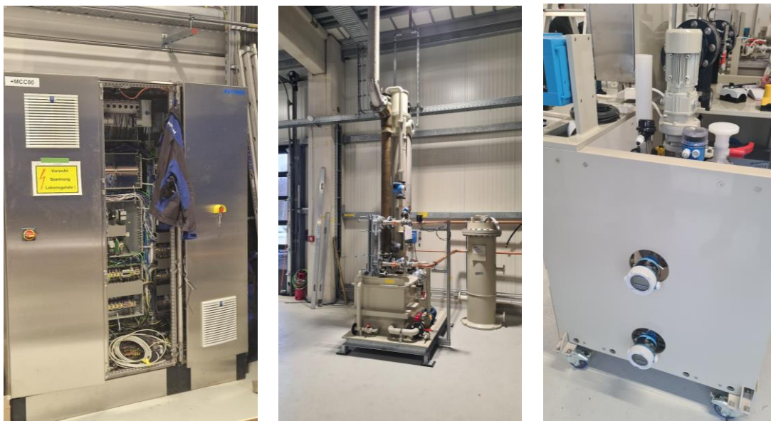
Figure 4 – Electrical Board and Various Equipment
