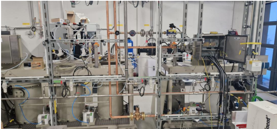
Figure 2 – Pilot Plant Vessels and Equipment
