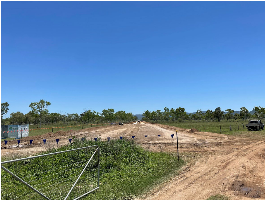
Figure: View looking north towards Jones Rd from QPM northern boundary – access road construction
