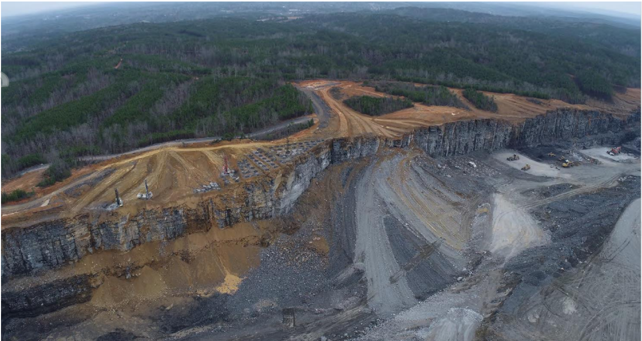
Image: Black Warrior Mine: new drills on top bench; D11T dozer push paths; benching to Newcastle seam; then to Mary Lee seam
