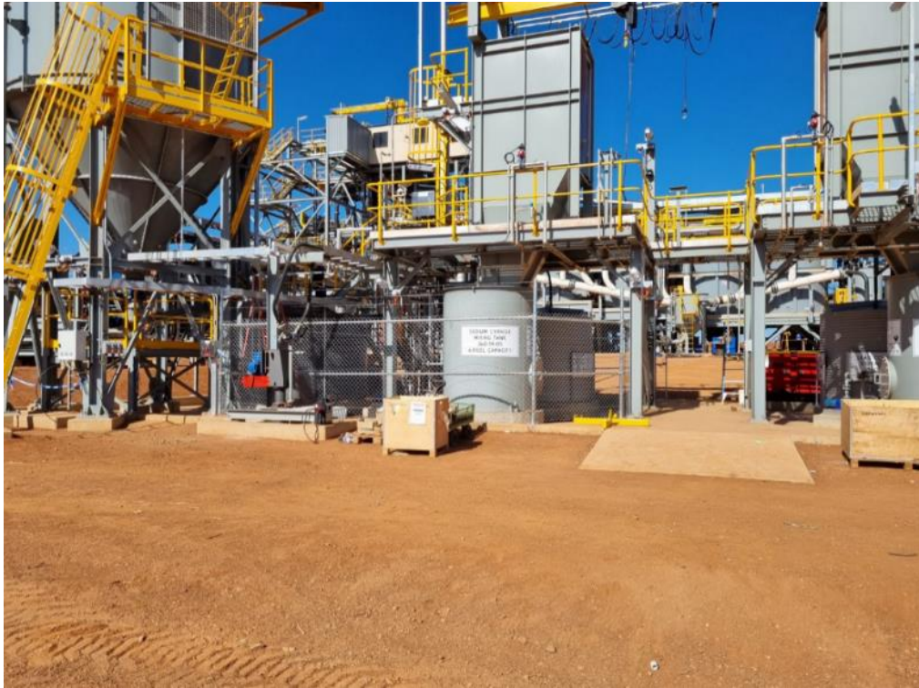
Figure 12 – Reagent mixing tanks (December 2022).
