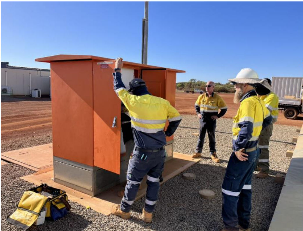
Figure 9 – Village permanent power connected (December 2022).
