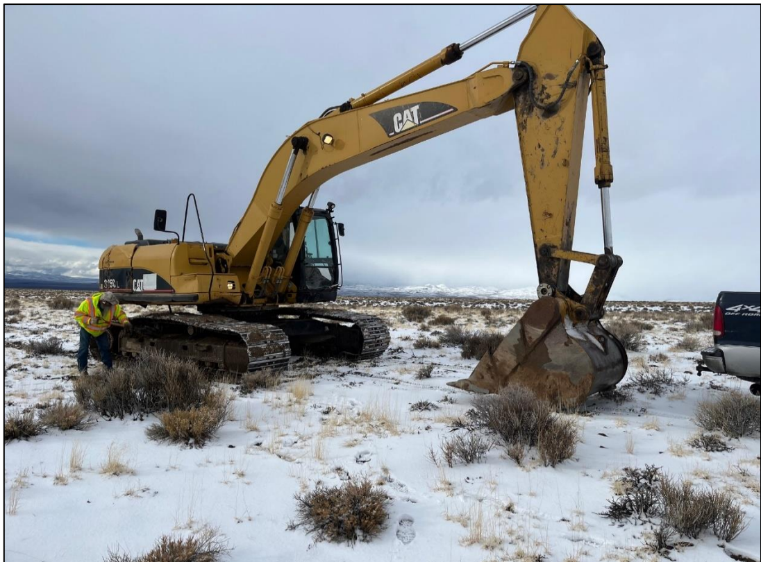
Image 2 – Clearing the drill pad after recent heavy snow at the Nevada Lithium Project (illustrating that the Project is accessible all year round)
